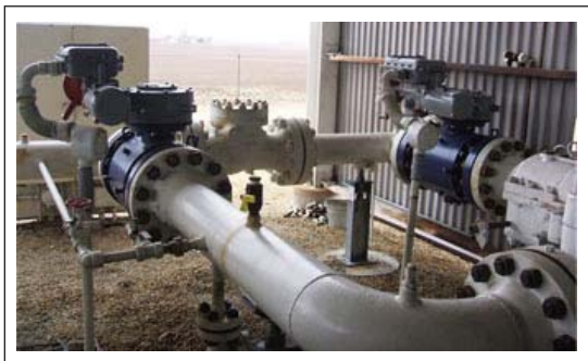
Crude Oil Pumping Station Pig Launcher/Receiver
