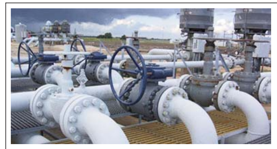
Salt Dome Brine & Gas Pumping Station
